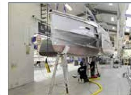
▲ After mounting the arms, the installation of the centreboard is part of the finishing touches.
